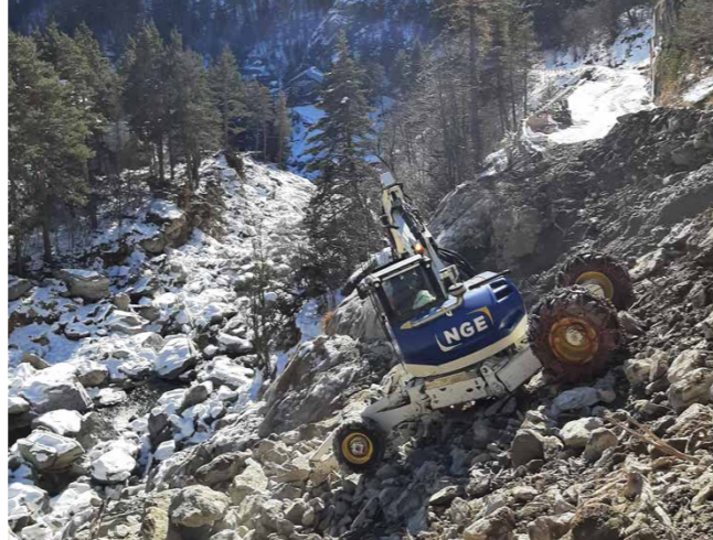
NGE at the bedside of the Roya Valley. Here, the spider excavator carries out the first surveys
